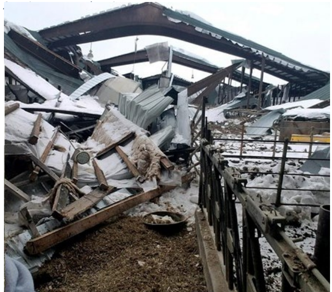
Figure 5 A Dairy Freestall Barn Collapsed due to excessive snow in 2019 in Olmsted County, MN.
